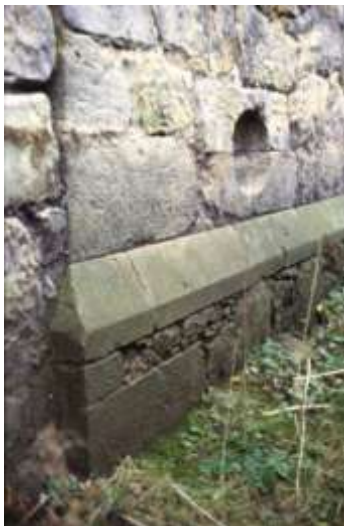
Illus 25: The chamfered plinth at the north-west corner of the tower with gun loop above. Looking SE.
